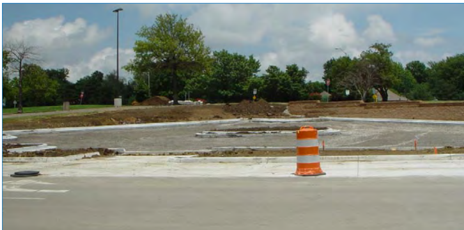
Future park-and-ride lot under construction (July 2011) at Oak Park Mall, near 95 th & Nieman (Northeast of the mall).
